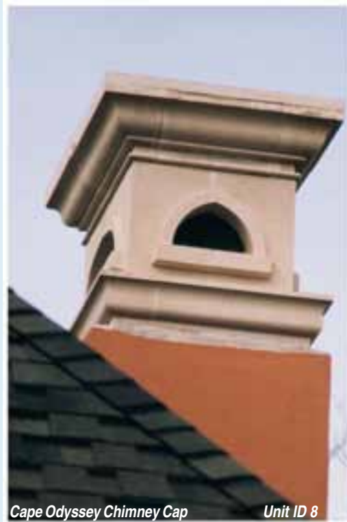
Chimney Cap using the Jamison2 and ThreeStep5 Profiles Refer to Chapter 9 - Profiles - The DNA of Stone for more Profile options
