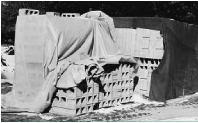
Figure 3. By placing masonry units on pallets and covering them with tarps, it is possible to keep them dry while stored at the job site. (29480-O)
