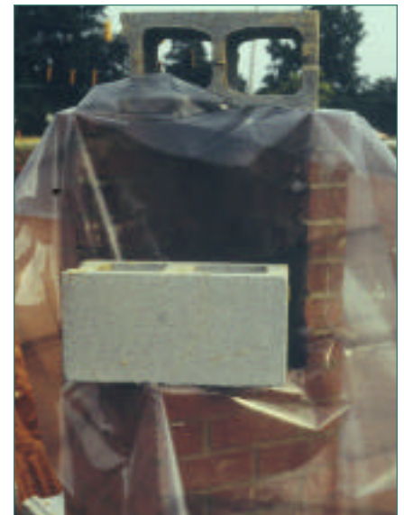
Figure 4. The top of masonry walls should be protected with a tarp whenever rain or snow is expected. It is good practice to cover work at the end of each day to help keep excessive water out and aid curing. (70028)
