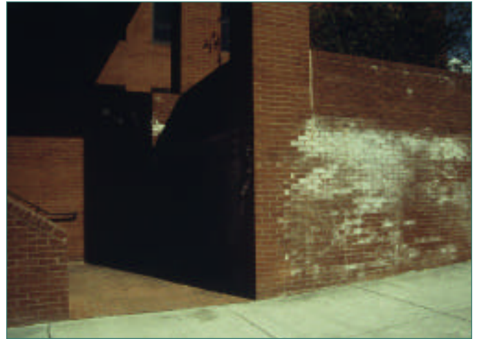
Figure 1. Efflorescence is often called "new building bloom" because it appears on fresh masonry surfaces. (70026)
