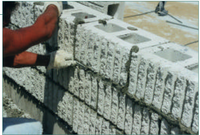
Figure 2. Tooling joints compacts the mortar and creates a weather-tight bond. This minimizes water entry into the wall, which reduces the potential for efflorescence. (70027)
