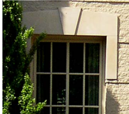
Exapmle of a Flatface Keystone Plinth blocks in the Circle Top Window surround.
