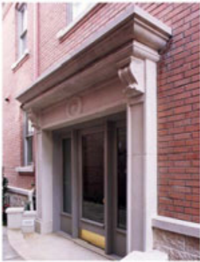
Note the Recess Pilasters on Plinth Blocks and Brackets below the Lintel
