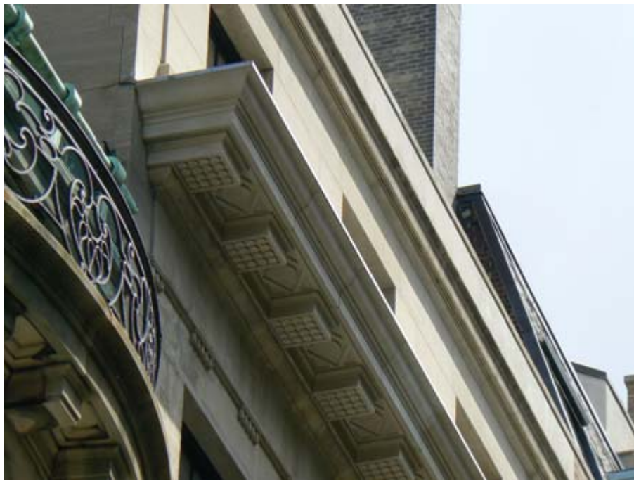
Towne House Restorations replaced a gravity loaded limestone cornice with this GFRC version in New York City.
