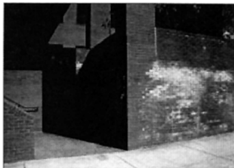
Figure 1. Efflorescence is often called "new building bloom" because it appears on fresh masonry surfaces. (T0026)
