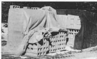
Figure 3. By placing masonry units on pallets and covering them with tarps, it is possible to keep them dry while stored at the job site. (20480-C)
