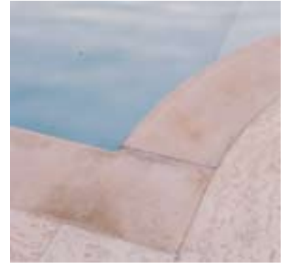
EXAMPLE PHOTO OF POOL COPING
