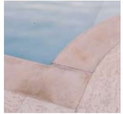
EXAMPLE PHOTO OF POOL COPING
