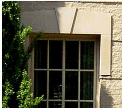
Exapmle of a Flatface Keystone Plinth blocks in the Circle Top Window surround.
