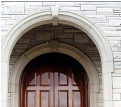
Note the wider Chamfer Keystone on the Circle Top Door surround in comparison to the one on the front of the building
