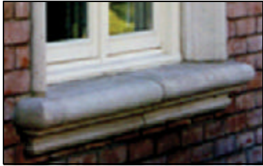
EXAMPLE PHOTO OF SILLS
