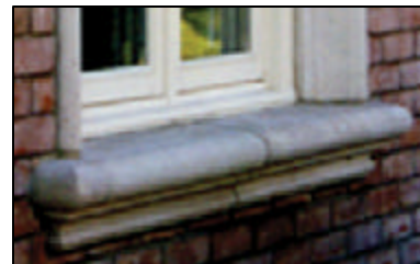
EXAMPLE PHOTO OF SILLS
